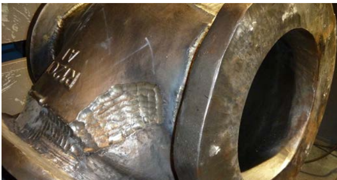
FOXcore 2594-T1 HD used for the repair welding of cast superduplex stainless steel.
