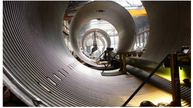
Welding of limpet coils with Ø 1.2 mm using FOXcore 316L-MC. Courtesy: Neuman Anlagentechnik, Germany
