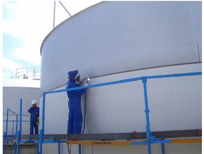
Welding on-site of stainless steel tanks – a typical application of Böhler Welding rutile all-position flux-cored wires. Tanks made of UNS S32101 and welded with FOXcore 2307-T1.
