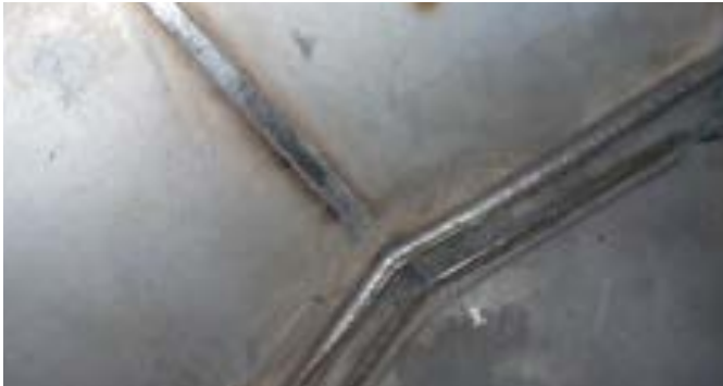
Welding of UNS S32205 in vertical-up and overhead position, using FOXcore 2209-T1.
