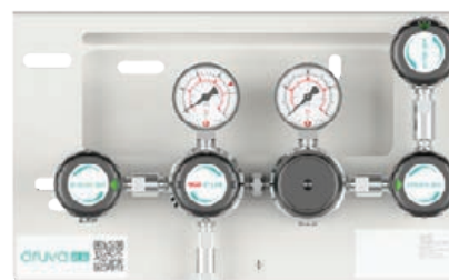
PS0 Inlet Tee Purge & Outlet Shut-off
