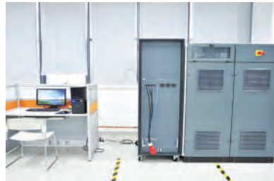
Harmonics & Flicker Test Laboratory
